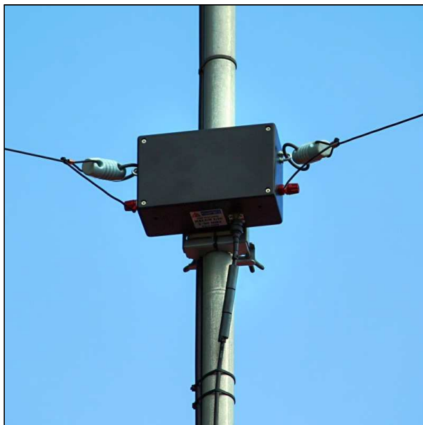
Balun box in 9 meters height, apex angle 80°
